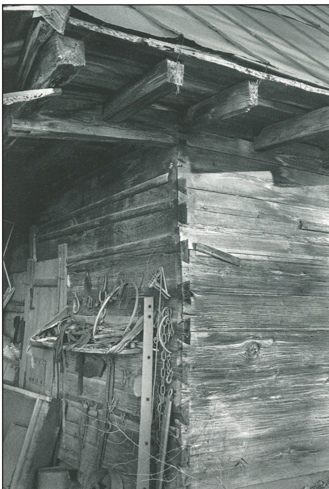
Photograph 6: Detail of dovetail plank construction on the Daniel Stone House. (Source: North Carolina Architecture p.177)
